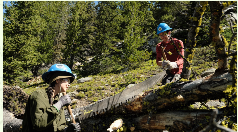
Trail maintenance on the Pacific Northwest Trail featuring PNTS Trail Intern, Evan Watson Photo Credit: Pacific Northwest Trail Association
